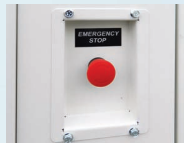
5 Emergency Stop Button
